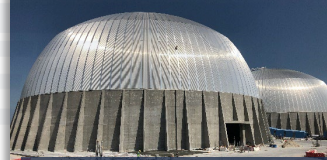
Aluminum Domes, KIPIC Refinery D = 87m, Al-Zour, Kuwait
